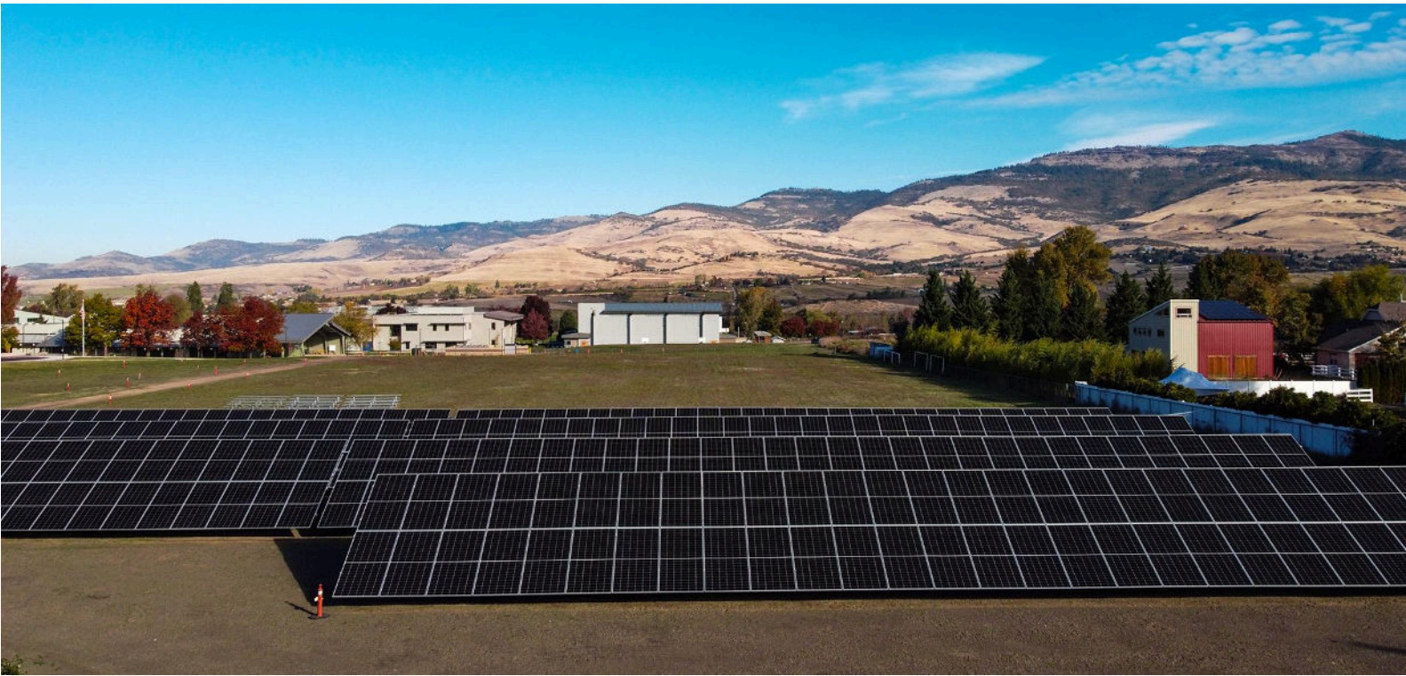
A 200 kW ground-mounted solar array at Ashland Middle School, installed in 2023.
