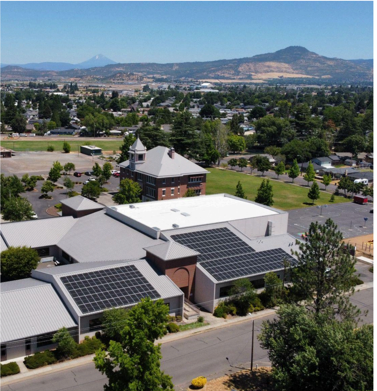
In 2024, True South Solar installed a 109 kW solar array atop Central Point Elementary School along with a 250 kWh battery backup system as part of a community resilience project funded by the State of Oregon.
